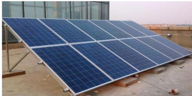
Figure 1. 5kw off grid solar panel
